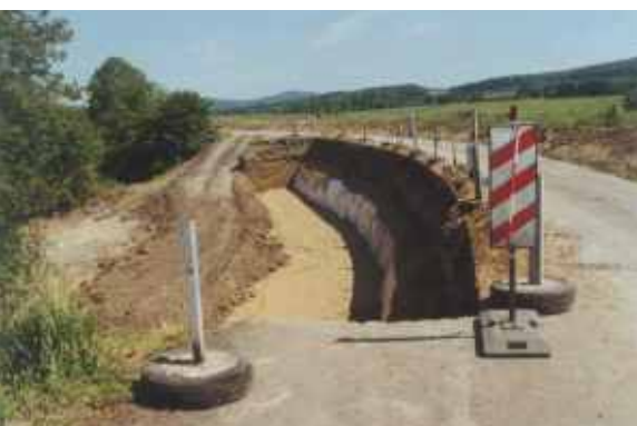
The landslide-deformed section of the road excavated down to the stable ground
