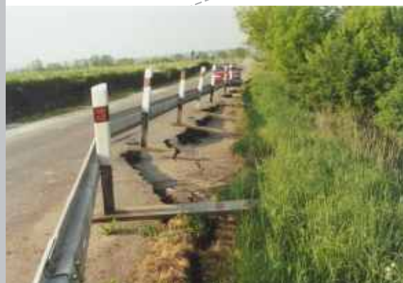
The road near Býčkovice destroyed by landslide (1999)
