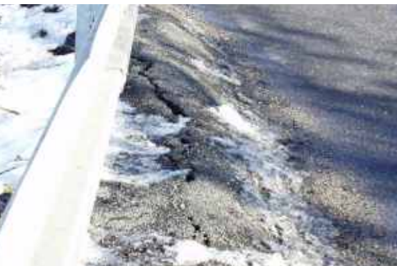
The road destroyed by landslide
