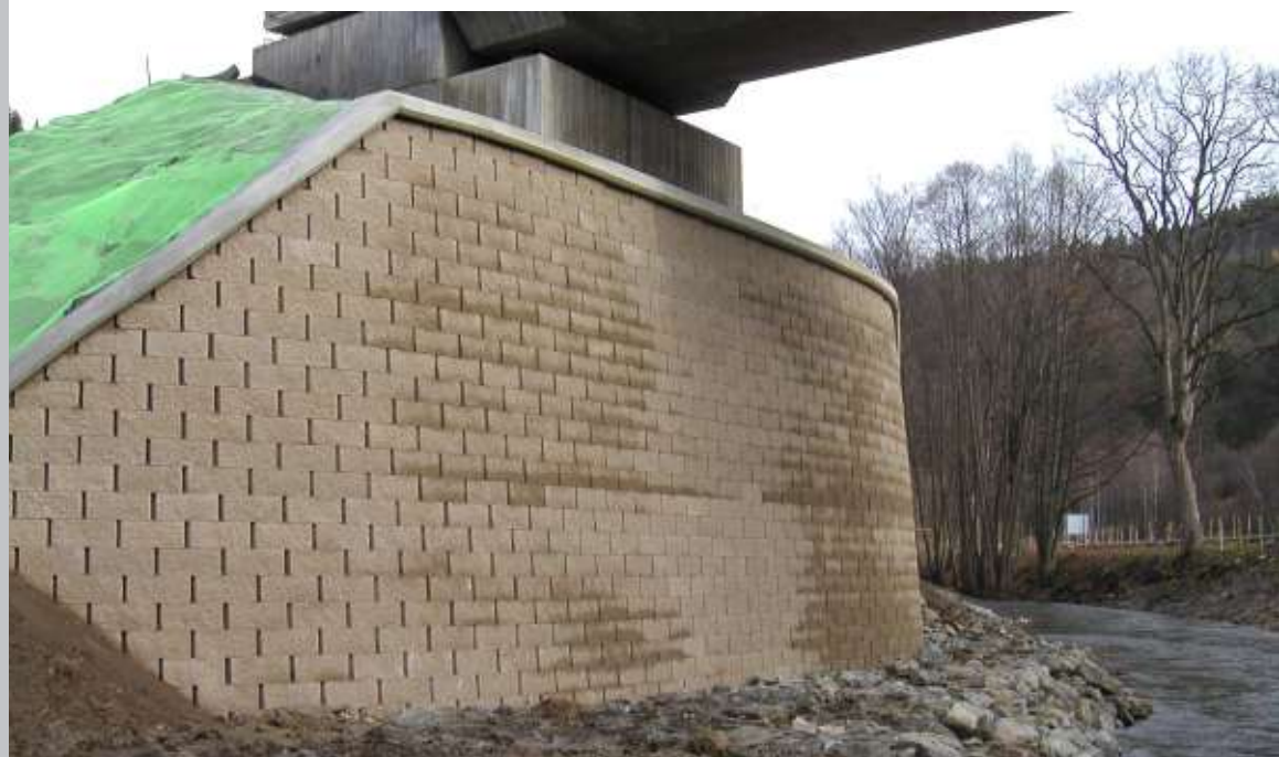
Completed bridge abutment made of reinforced soil. The side slope surface is reinforced with Slovarm geotextile to ensure erosion control.
