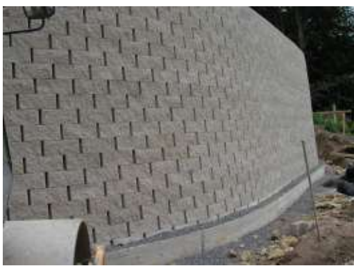
View of the segmental wall of a bridge abutment on the building site.
