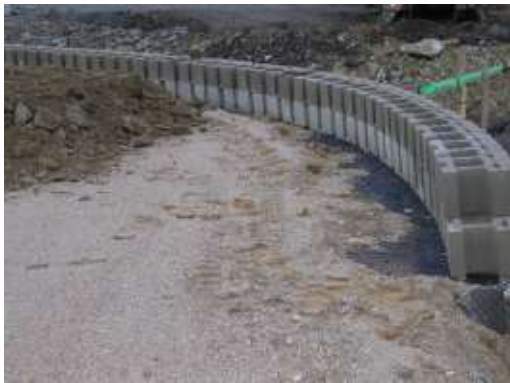
Detail of face segments laying (adapting pieces). The reinforcing geogrid Armatex® G 55/30 is inserted into the horizontal joint of every other layer.
