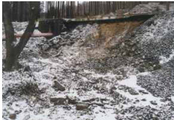
Fig. 2 View of slide of road from storage area
